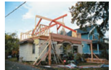
Main rafters starting to take shape, new street level porch header in place.
