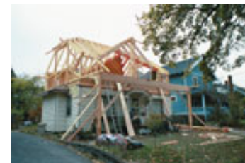
With most of the roof rafters in place we can now start to see the roof line.
