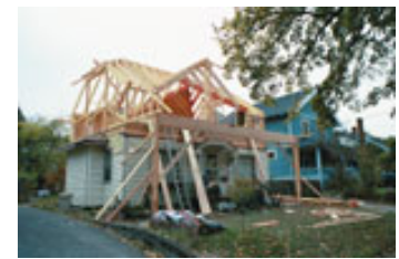
With most of the roof rafters in place we can now start to see the roof line.
