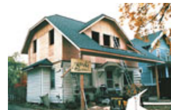
With the new roof installed, and exterior framing of the second story done, you can now see how the second story porch will be integrated into the design.
