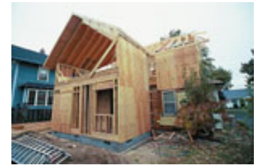
View of the new small addition at the back of the house. On the first floor a bath and extension to the dining room, on the second floor a sitting room off the master bedroom.
