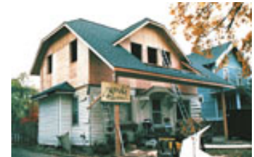
With the new roof installed, and exterior framing of the second story done, you can now see how the second story porch will be integrated into the design.
