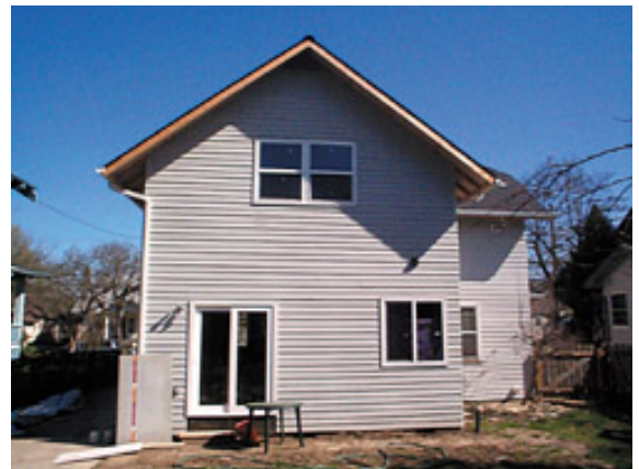
150 sq ft addition includes a new bathroom, kitchen expansion, and second-story sitting room.
